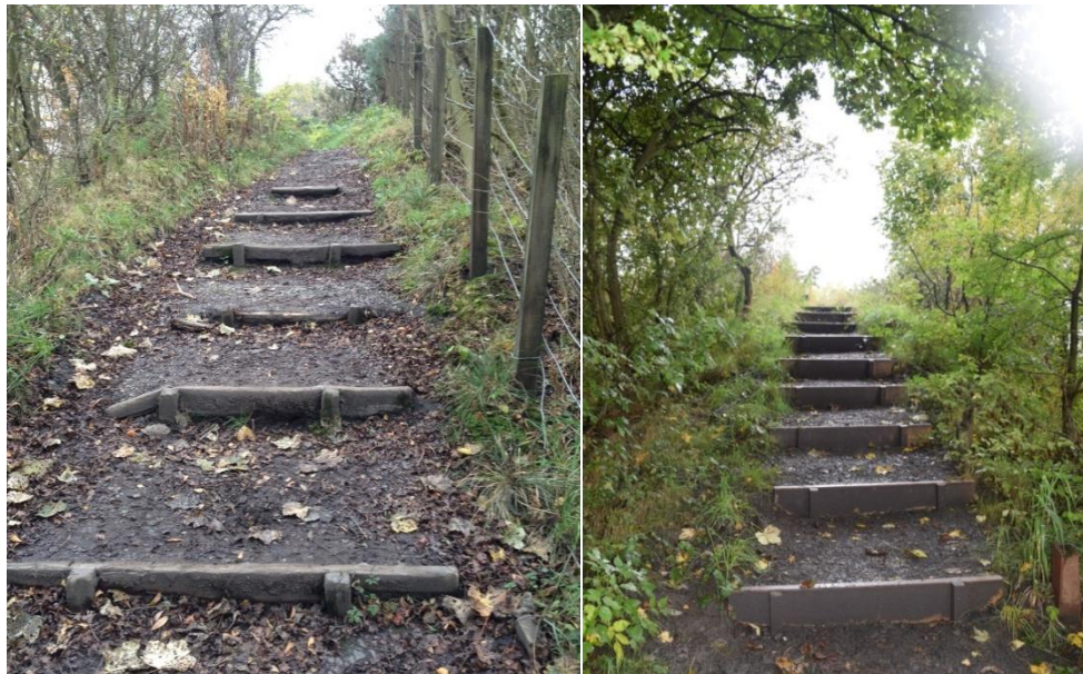
Bing on south shore – steps needing repair (left) and steps that have had repair by Paths for All and Education Community Learning and Development project (right).
