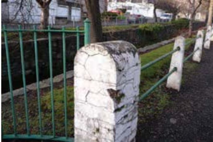
Public realm in some place appears tired and neglected
