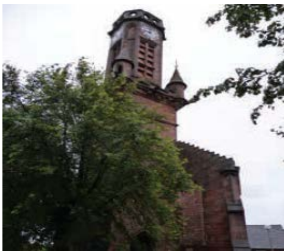
The Clock Tower is in need of repair and maintenance
