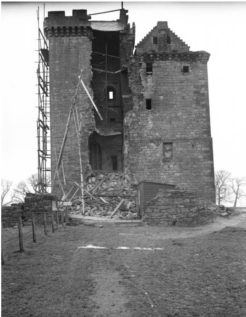
Figure 4-21: Clackmannan, Clackmannan Tower collapse in mid 1940s (© RCAHMS)
