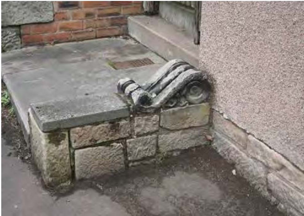
Figure 4-12: Clackmannan, 42-44 High Street, August 2014 – recycled ornamental scroll bracket detail (Peter Drummond Architects)
