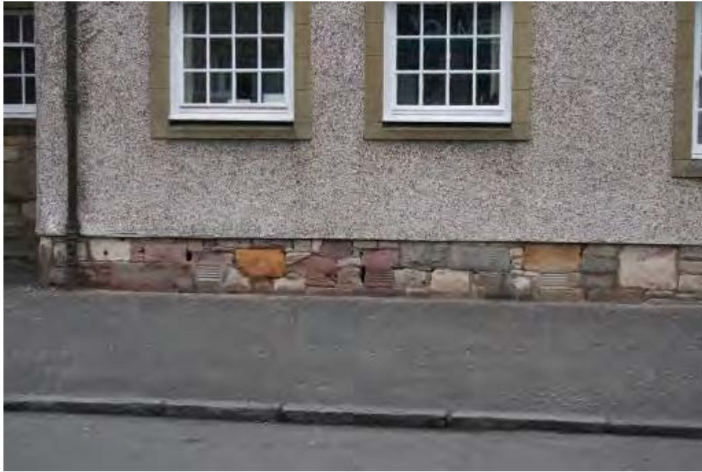
Figure 4-11: Clackmannan, 33-39 Main Street, August 2014 – weathering of stone base course (Peter Drummond Architects)
