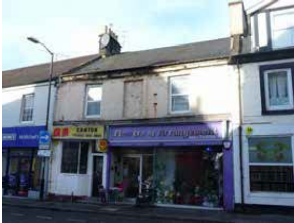
Above: Nos. 11-13 Mill Street is in poor condition.
