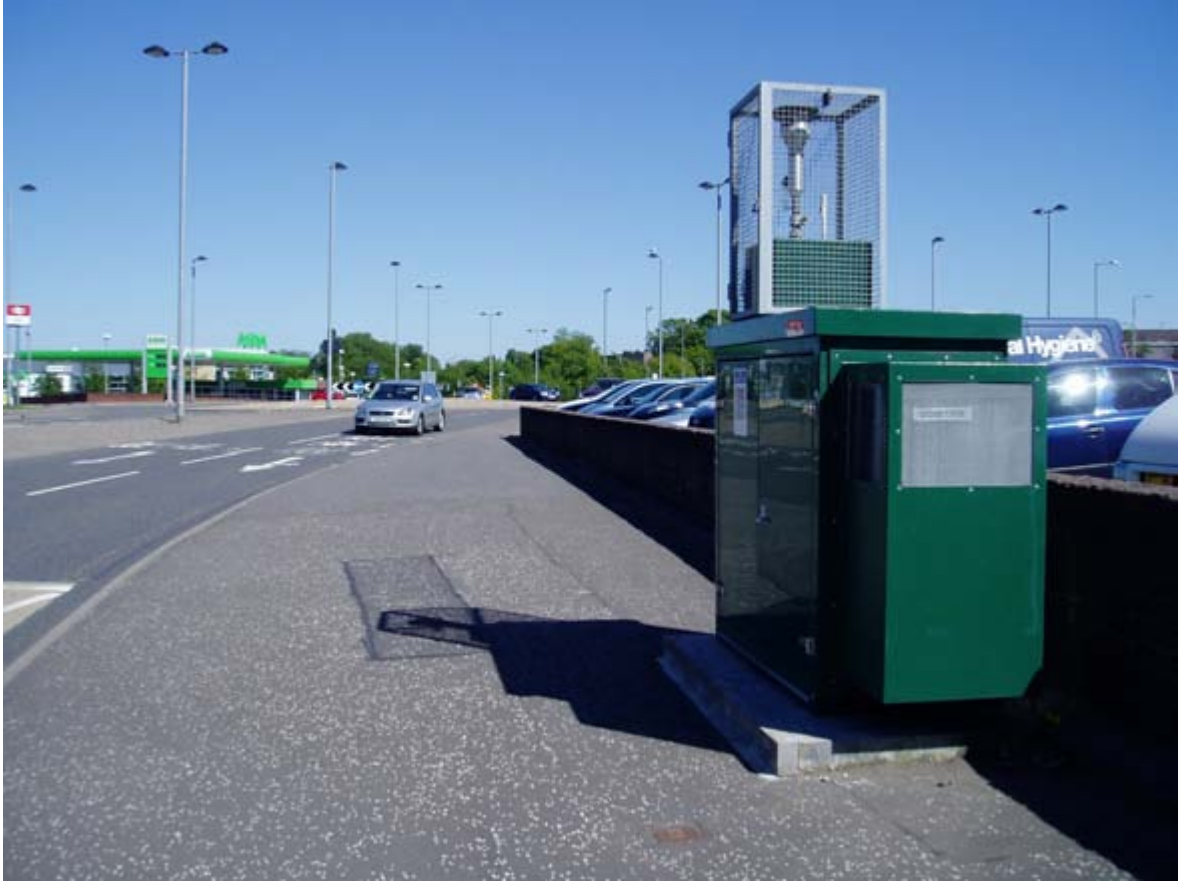
Figure 2.1 Photograph of new FDMS Automatic Monitoring Site at South Ring Road, Alloa
